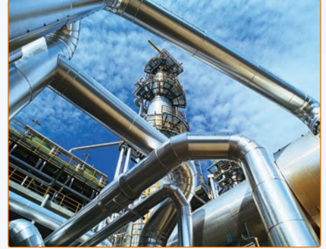
Chemical, Oil and Gas
